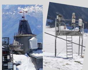
Abb.2: TAWES am Sonnblick Observatorium Fig.2: TAWES at the Sonnblick Observatory Quelle/Source: ZAMG
