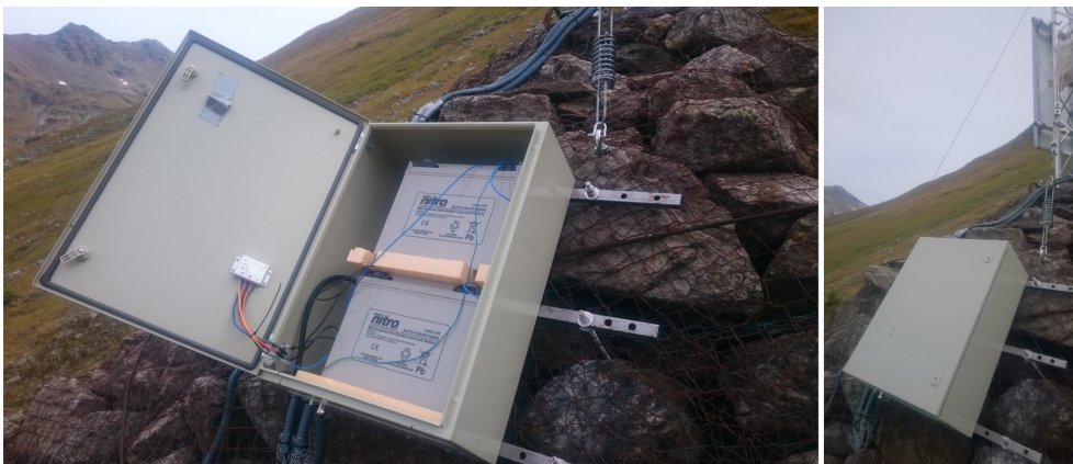
Figure 3.33: In autumn 2019, a new battery enclosure was mounted. The new enclosure hosts two batteries providing a total capacity of 3240 Wh.
