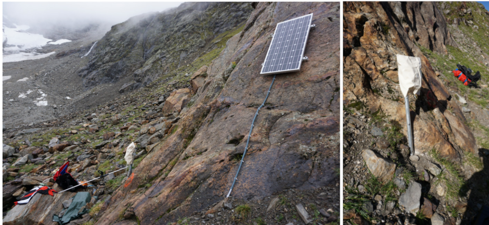
Figure 3.36: The first version of the PIL station. The solar panel was mounted on a southeast-facing rockwall in a height of about 3 m above ground. The Ruwai data recorder was mounted on a ~1 m mast. The battery box is placed below the mast base.
