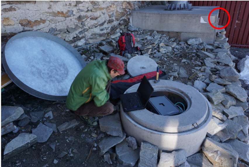
Figure 3.21: GPS signal tests after the OBS station installation. The GPS antenna (red encircled) was initially mounted on the close by wind tower foundation.
