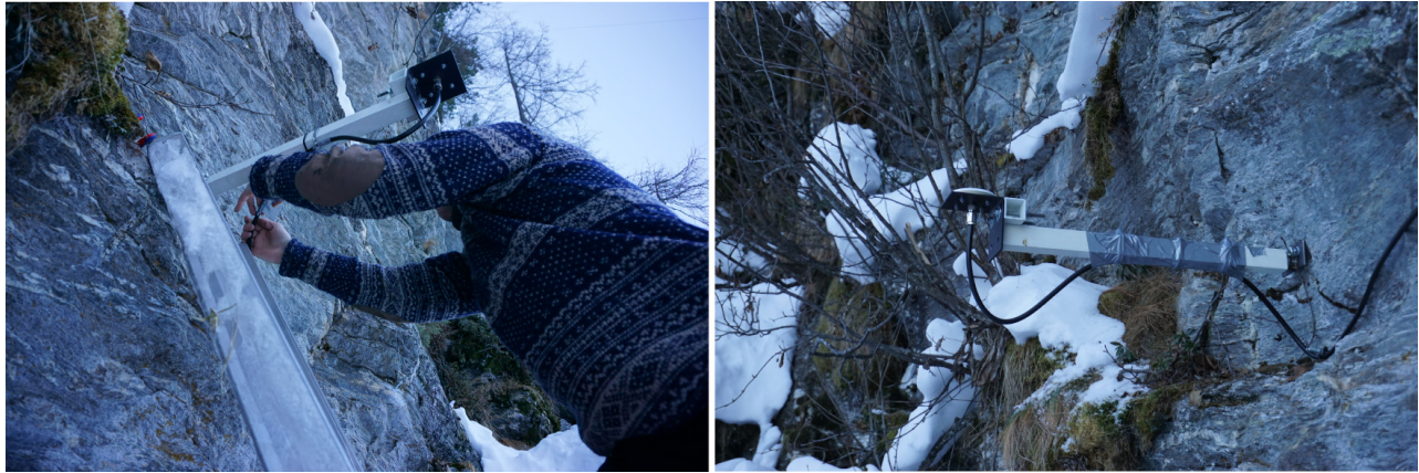
Figure 3.25: Originally, the GPS antenna was mounted directly on the rockwall. In January 2017, a \sim 0.5 m beam was mounted to raise the antenna's sky view percentage which substantially improved the GPS signal strength.
