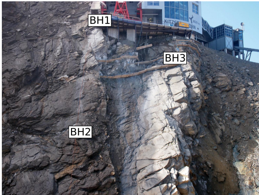
Figure 3.44: SeisRockHT investigation site at the north-face below the Kitzsteinhorn cable car top station. Deep boreholes 1 (BH1) and 2 (BH2) are normal to the local surface which results in a borehole inclination of about 40^\circ . The 6 m deep borehole 3 (BH3) is vertical (borehole inclination 0^\circ ). All boreholes are drilled into solid rock.
