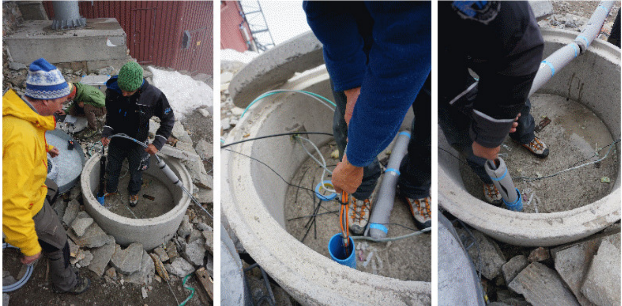
Figure 3.20: The OBS three component seismometer is sunk in the 21 m deep BH1. The sensor is situated at the lower end of a thermistor string.
