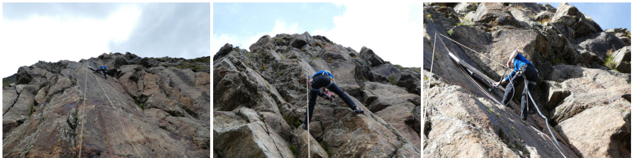
Figure 3.39: Installation of the solar panel power cable in late summer 2017.
